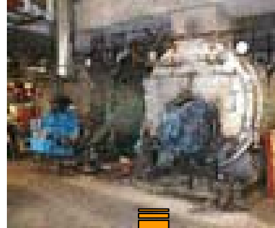
C&I High Efficiency Heating Program
