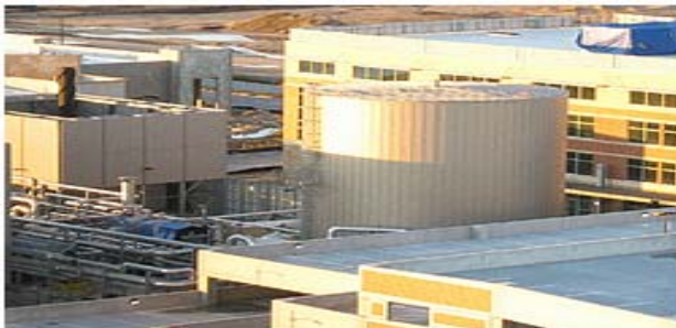
Steel Tank of the Year - Special Storage Dell Children’s Medical Center in Austin, TX Built by CB&I Constructors Inc., The Woodlands, TX
