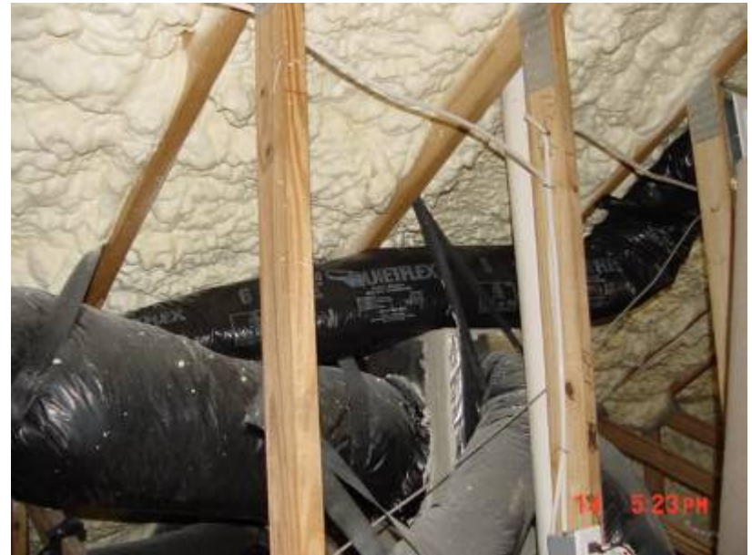
Ducts in conditioned space
