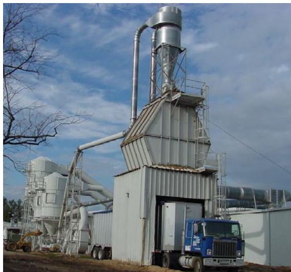
Figure 4. Photograph of a Typical Dust Collection System
