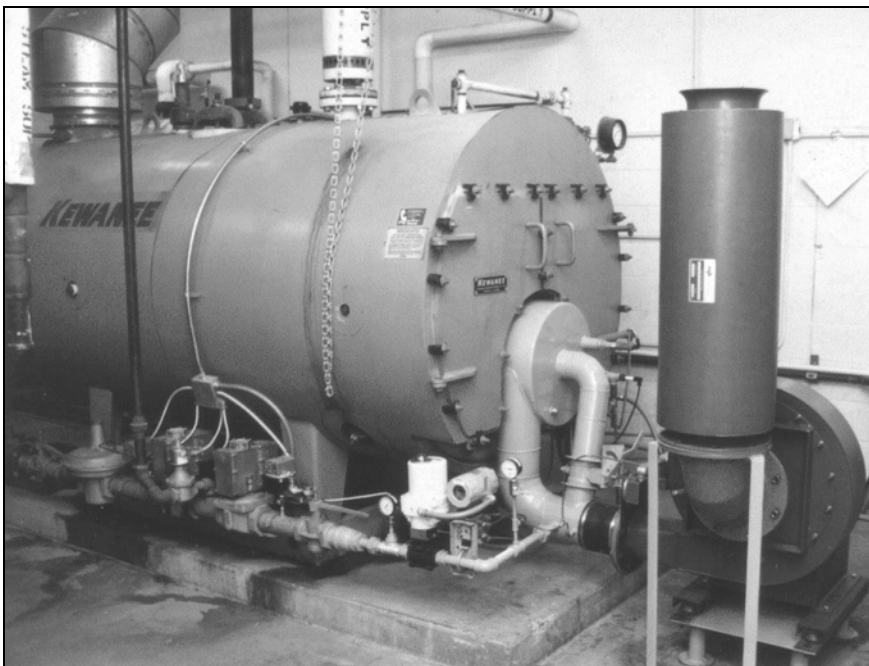
Figure 4. 2.5-Million-Btu/h FIR Burner Installed on Vandenberg AFB Firetube Boiler
