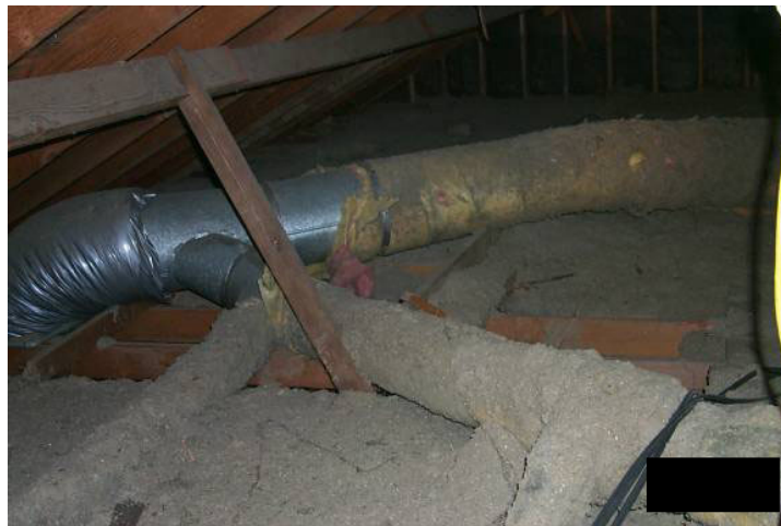
Figure 2. Poorly Insulated Sheet Metal Ducts and Blown-In Insulation in the Attic before Retrofit
