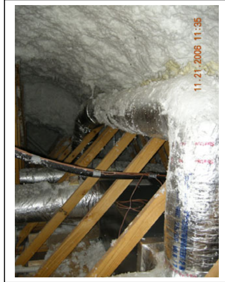
Figure 2. Three Ton HVAC Unit in the Conditioned, Sealed Attic
