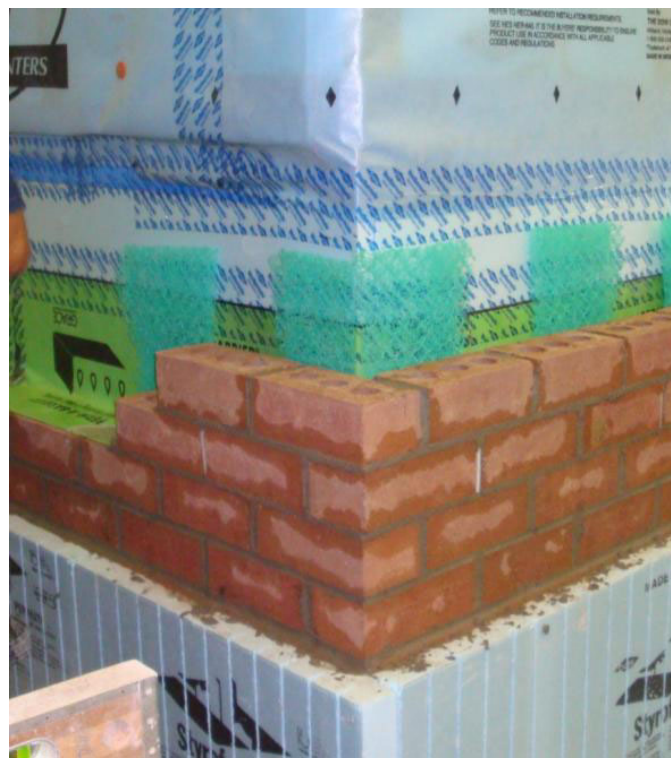
Figure 2. Foundation Wall Mock-up Highlighting Integration with Above-Grade Wall and Through-wall Flashing and Polypropylene Net Material Product at Brick Detail
