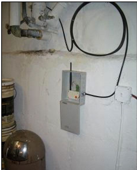
Figure 3. Cable Interconnects and Network Node
