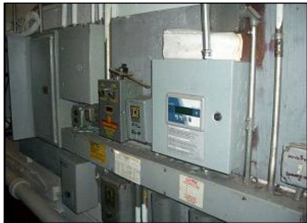
Figure 6. Replacement Heat Controller
