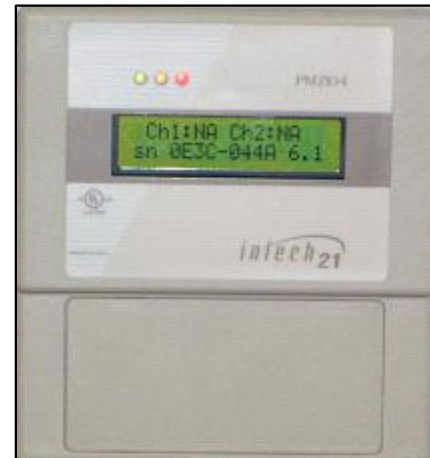
Figure 7. Typical apartment submeter with LED lights
