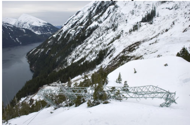
Figure 2. A tower on the Snettisham transmission line destroyed by avalanche
