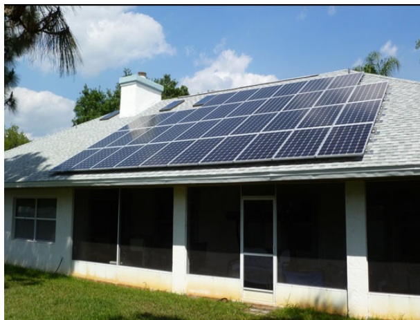
Figure 13. 10 kW West-facing PV system installed at Site 19.
