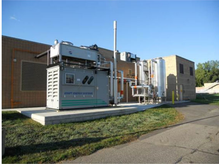
Figure 5. Biogas Fueled Electric Generator
