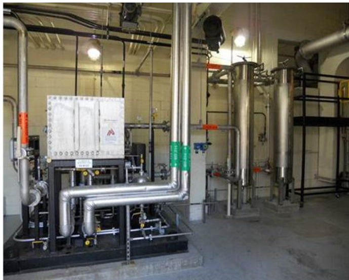
Figure 2. Biogas conditioning system
