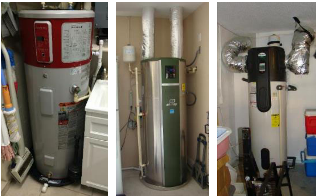
Figure 4. HPWH configurations: Left, interior GE unit in utility room, Site 13; center, ducted Airgenerate unit at Site 5; right, ducted A.O. Smith unit at Site 26.
