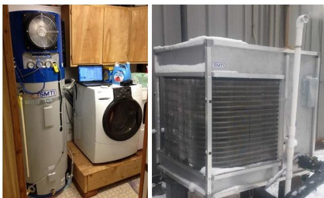
Figure 1. GHP as Water Heater (Left) and Space Heater (Right) Units in Field, in WA and TN
