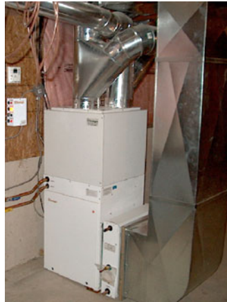
Figure 6. Zoned forced air, combination space and water heating system. Source: Natural Resources Canada, 2015
