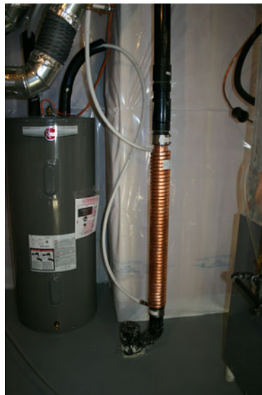
Figure 5. Drain Water Heat Recovery unit installed in a LEEP field trial home. Source: Gary Proskiw, 2015
