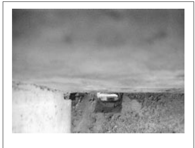
Figure 4. Typical floor penetrations for radiator pipes; note also grouted notch to the left.
