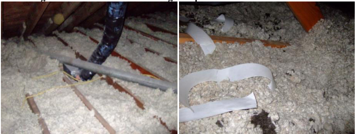
Figure 3. Attic Insulation Showing Compressed and Inconsistent Fill
