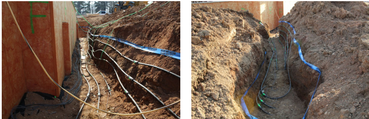
Figure 4. FHX in basement wall excavation (Left) and HGHX in utility trench (Right)
