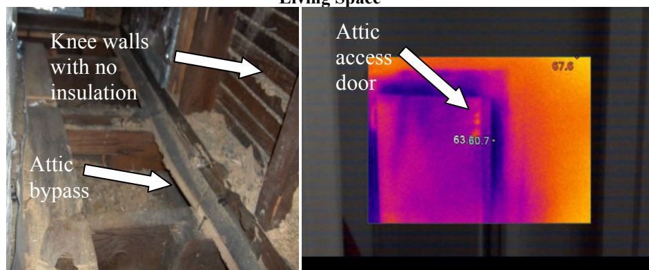
Figure 4. Attic Bypasses. Picture on the Right is a Thermal Image of the Attic Access Door Taken in the Winter while the Home was Depressurized. The Blue Color in the Image Shows Attic Air Infiltration into the Living Space
