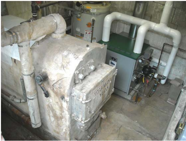
Figure 4. Existing Low-Pressure Steam Boiler (left) New Low-Pressure Steam Boiler (Right)
