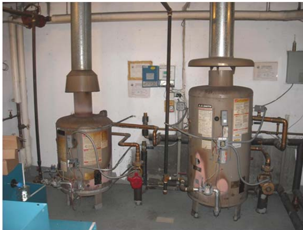
Figure 6. Existing Water Heaters
