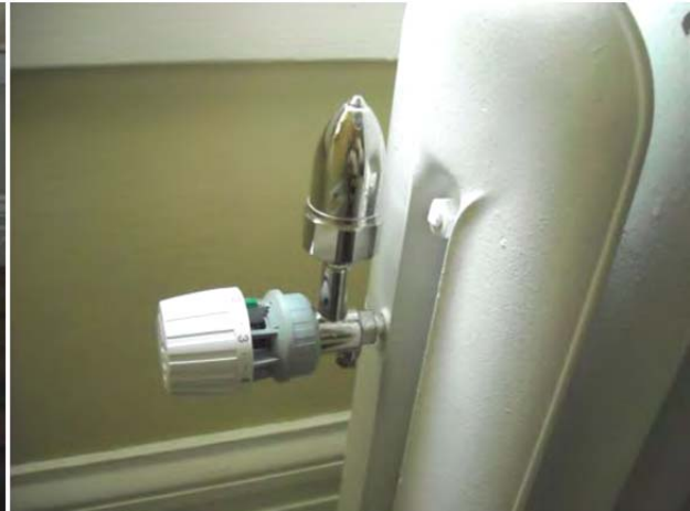
Figure 9. Close up Photo of TRV with Air Vent
