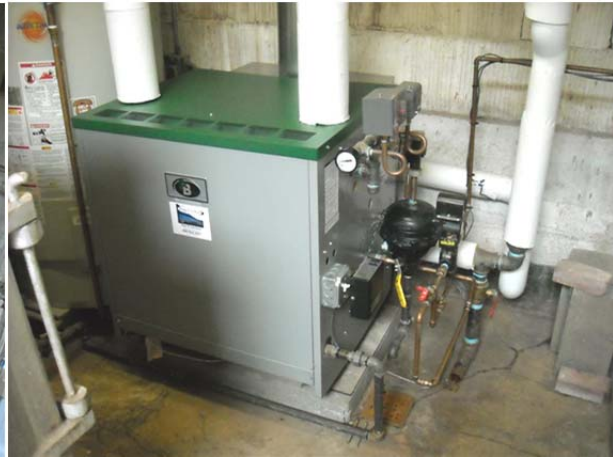
Figure 5. New Low-Pressure Steam Boiler (close up) New Hot Water Heater in Corner
