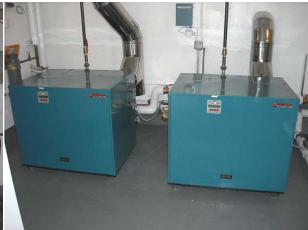
Figure 7. New High Efficiency Water Heaters
