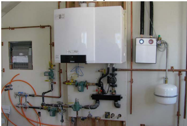
Figure 3. A 95 Percent Energy-Efficient Boiler Piped to a Low Temperature Radiant Heat Flooring System
