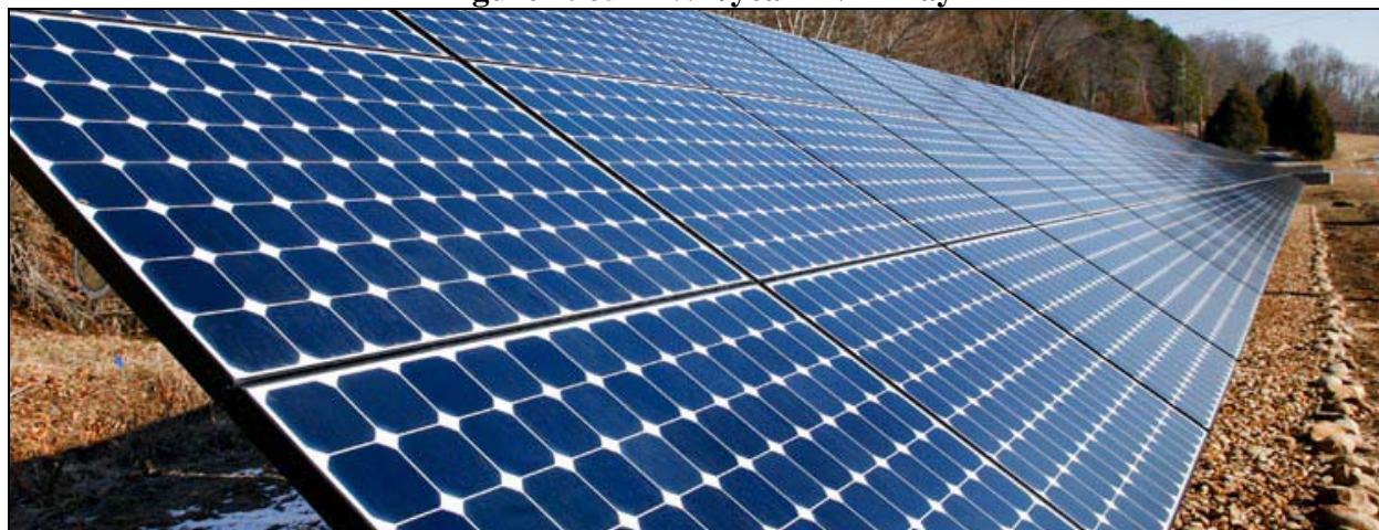
Figure 4. 65-MWh/year PV Array
