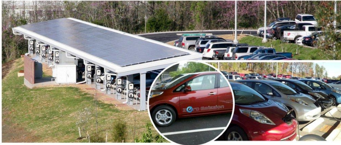
Figure 7. Electric Vehicle Charging Station
