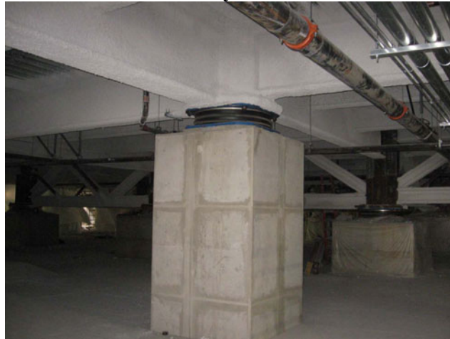
Figure 1: Typical Base Isolation Seismic System Used in the Pacific NW Test Hospital
