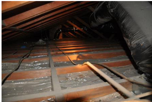
Figure 3. Grange 1948 attic accordion foil insulation and long HVAC return system strapped to rafters. Source: R. Chitwood, pers. comm., 2012.
