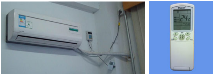
Figure 7 Typical room air-conditioning at home and controller
