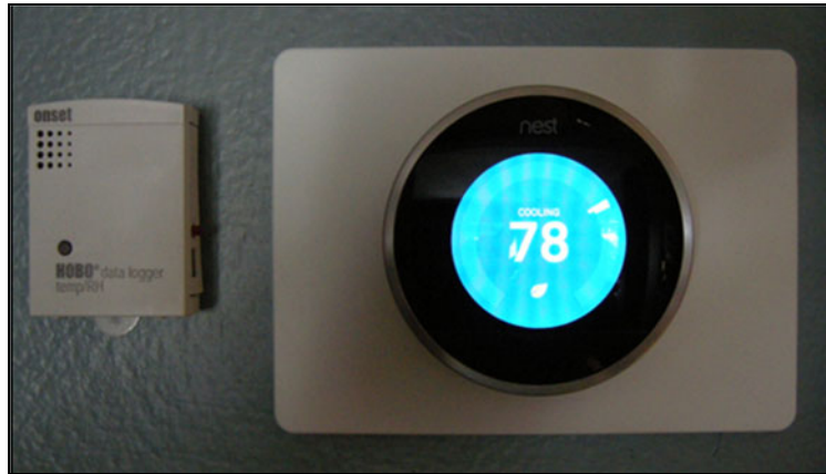
Figure 1. The Nest learning thermostat installed at one of the PDR sites showing portable logger recording temperature/humidity right by original thermostat & smart replacement.
