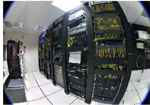
Inside a data center
