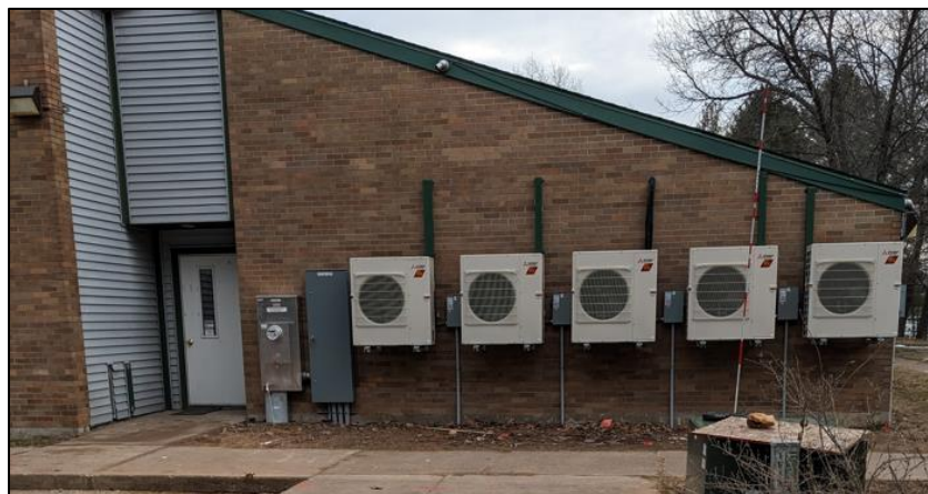
Figure 3: Photo of air-source heat pump air handlers installed at the Elk Point West apartments in Lac du Flambeau, WI. Source: Elevate
