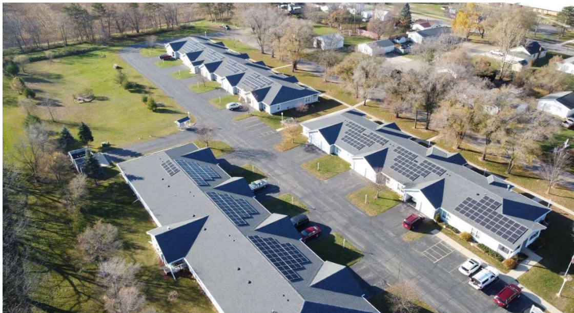
Figure 1. Brodhead Senior Village 106 KW solar installation. Source: Midwest Solar Power LLC
