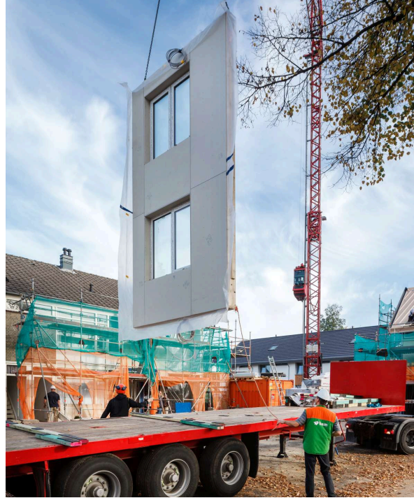
Figure 2. A wall and window retrofit panel being lifted from a truck bed by a crane. Source: RMI 2022.
