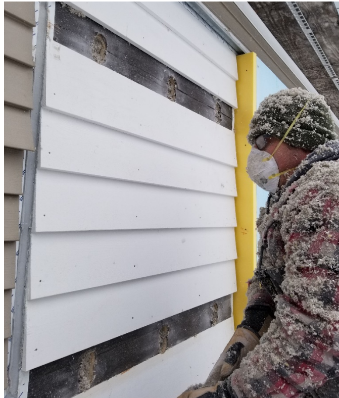
Figure 1. An insulation contractor inspecting a drill-and-fill insulation retrofit installed in an experimental facility. Source: Patrick Huelman, University of Minnesota
