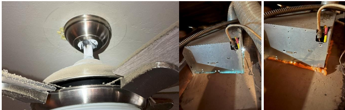
Figure 6. Photo of sealant buildup on ceiling fan (left), and foam applied around bath fan housing (middle and right)
