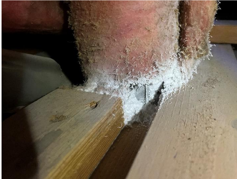
Figure 8. Sealant deposition on ductwork at register boot connection
