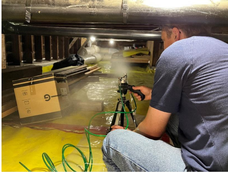
Figure 5. Aerosol sprayer setup in crawlspace at Site 2. Water is used to check functionality before injecting sealant.
