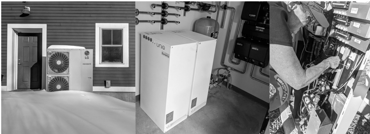
Figure 3: Photos of Type 4 system installed for pilot study in Massachusetts (CZ 5a/6a)
