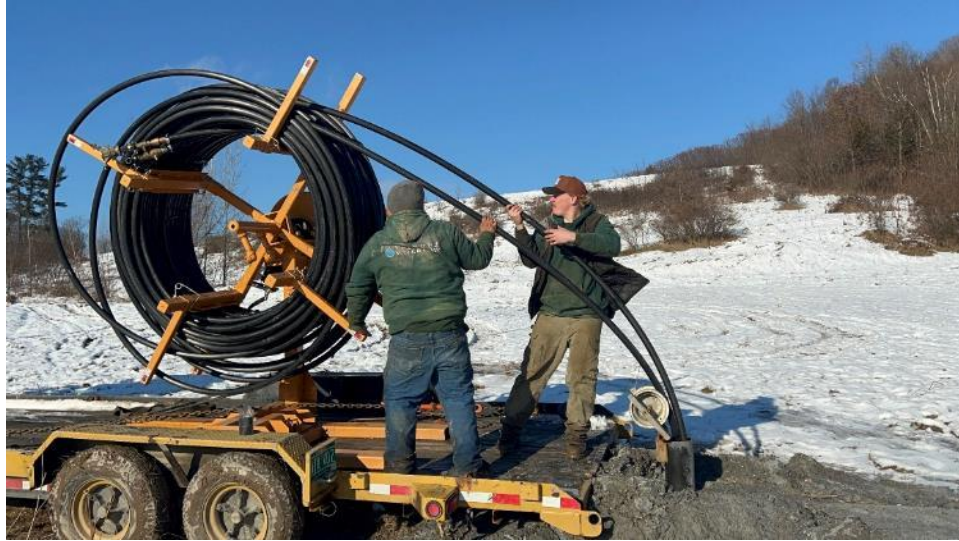
Figure 2. Polyethylene pipe being inserted in the borehole creating during construction of the borehole heat exchanger used for the thermal response test.
