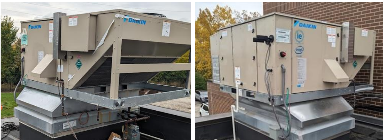
Figure 7: Daikin Rebel 4-ton Hybrid RTU demonstrations Source: GTI Energy
