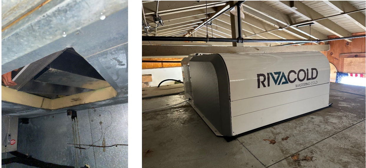
Figure 5. Image on the left shows the hole cut in the top of the walk-in from inside the cooler as the Rivacold unit is being set in place from above. Image on the right shows the fully installed unit on top of the walk-in.
