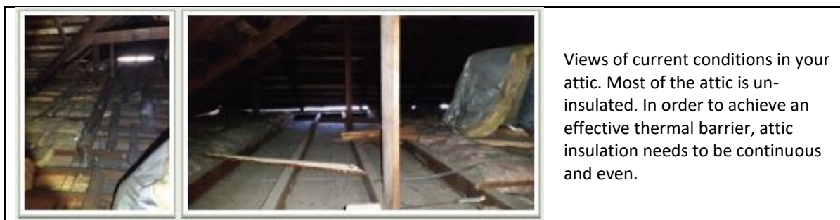
Figure 2. A good use of images, with clear photographs of the customer's home (rather than stock photos) alongside an explanation of the energy issue being depicted. Source: Assessment report by Hassler Heating and Air Conditioning.
